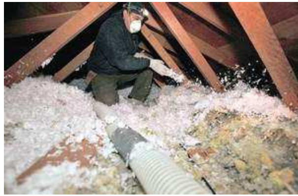
Subcontractor Abel Hernandez, 39, of Redmond, sprays fiberglass insulation in the attic space of Lona Hale’s northeast Bend home Thursday morning. Because of savings on her energy bills, the improvements should pay for themselves in five to seven years, according to GreenSavers’ Dave Bowman.
